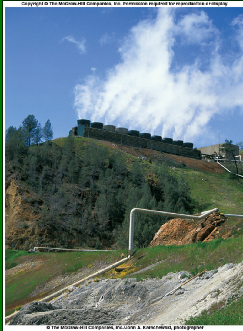
Geothermal power plant
