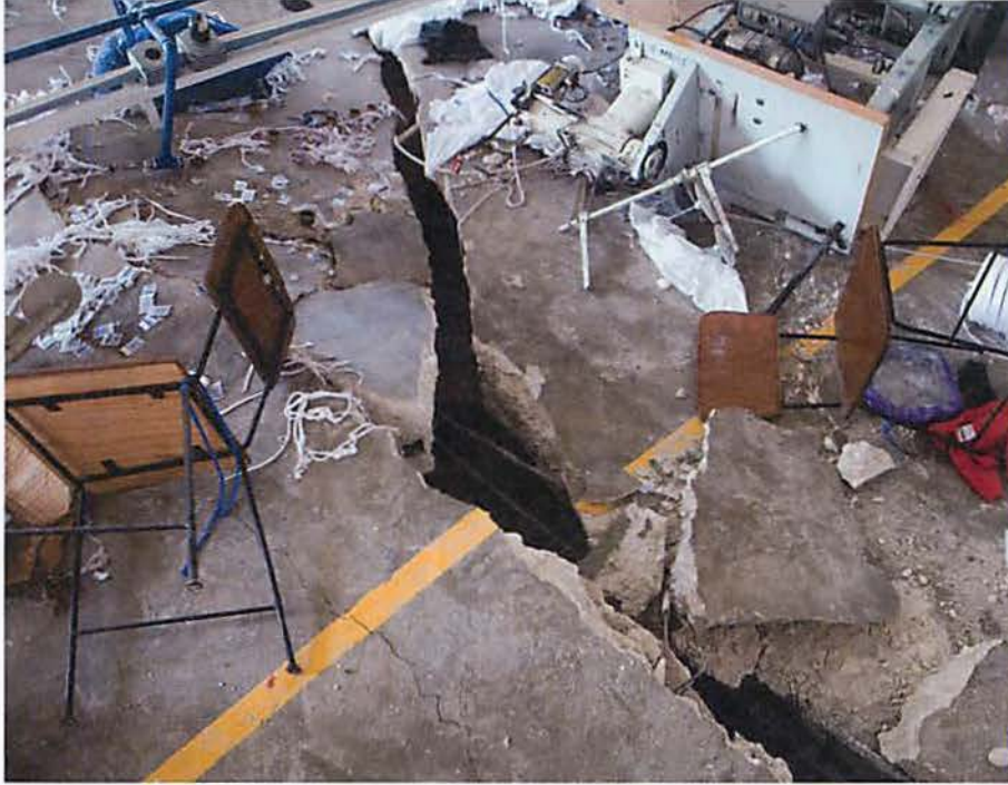
FIGURE 24.12 Earthquake damage in Haiti. The 2010 earthquake in Haiti killed more than 200,000 people and destroyed most of the structures in the capital, Port-au-Prince. (Dominic Nahr/Magnum Photos)
