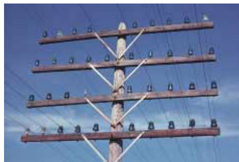
Electrical insulators on telephone poles are often made of glass because of its low electrical conductivity.
