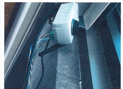
THE CONNECTING WIRES
